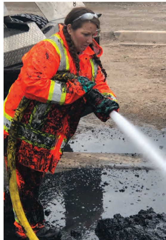
Julie General conducts remedial work, washing away contaminants that have met the soil and ensuring proper disposal of the hazardous waste.
